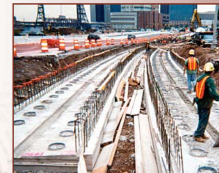
Final Design and Construction Assistance for the Newark-Elizabeth Rail Link First Operable Segment (FOS) - NJ Transit
