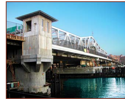
Construction Inspection for the Replacement of the Third Avenue Swing Bridge over the Harlem River - NYCDOT
