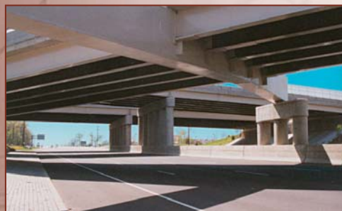
Construction Inspection for Route 1 & 130 / Georges Road Circle Elimination and Intersection Reconstruction - NJDOT
