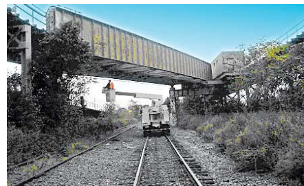
Comprehensive Assessment of Line Structures on the Bay Ridge & Bushwick Branches - MTA Long Island Rail Road
