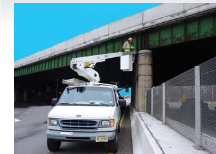
Biennial Inspection of Local & Arterial bridges in NY City & Upstate Regions - NYSDOT
