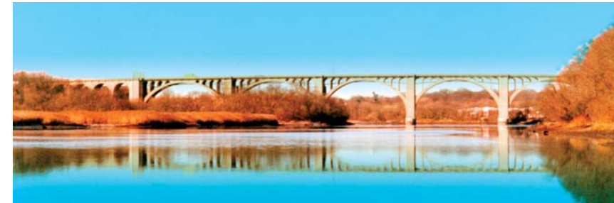
US Route 1 NB Bridge Over Raritan River, NJ NBIS Inspection of over 1000 Simple & Complex Vehicular Bridges throughout New Jersey - NJDOT
