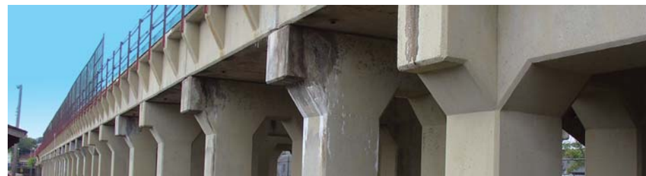
In-Depth Inspection of Bridges and Viaducts carrying Staten Island Rapid Transit - MTA / NYC Transit
