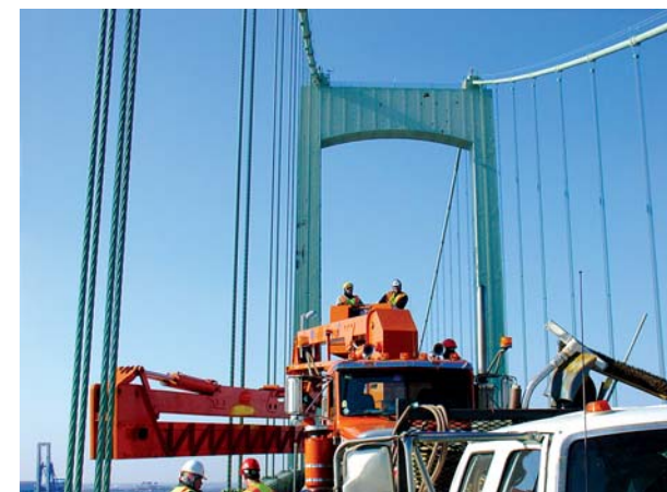
In-Depth Inspection & Deck Condition Assessment of the Walt Whitman Bridge Suspension and Anchorage Spans - Delaware River Port Authority
